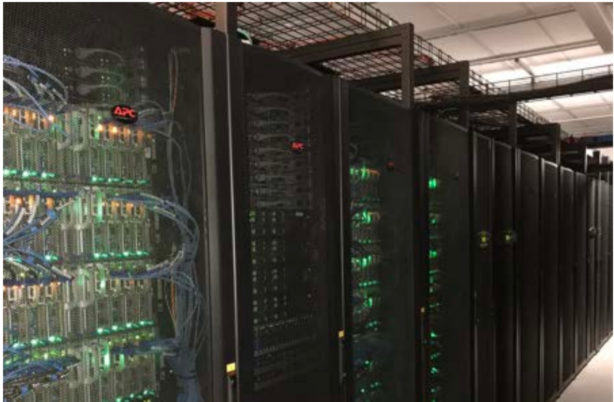
Above: One of many server racks at the National Computation Infrastructure, the site of NCIG computation and storage. Photo by J. Stenhouse
